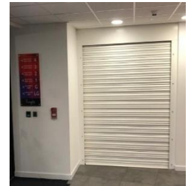
Tubular motor fire shutter Manchester University
