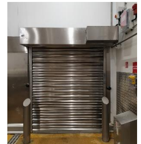
Stainless Steel fire shutter McDonald's Food Factory
